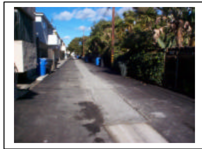
Figure 11. Porous concrete V-swale in a City alley to harvest runoff and reduce flooding of adjacent properties.
