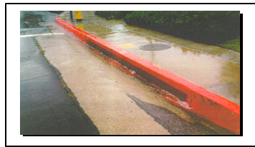
Figure 14. Catch basin screen operating during storm. Water can flow through the openings while keeping trash out.
