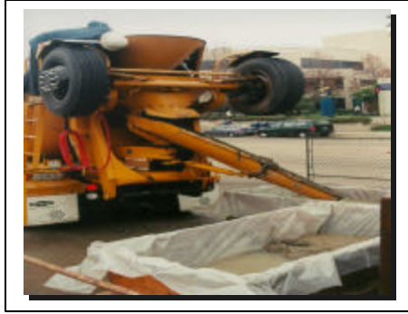
Figure 2. Concrete washouts are collected for disposal instead of released to the street, storm drain system and ocean.
