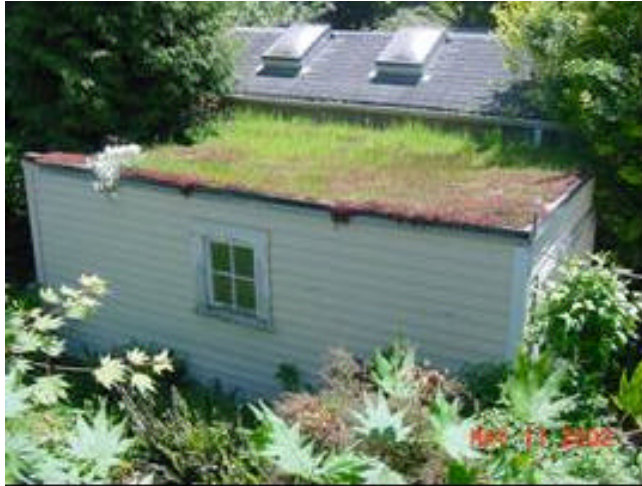
Figure 3. View of a residential garage EcoRoof that was monitored for a two-year period.
