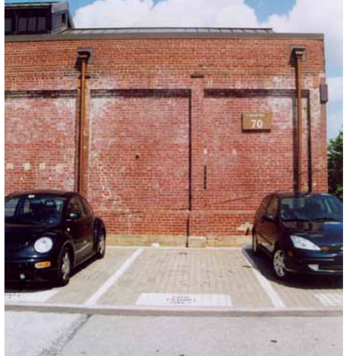
Above: Permeable parking spaces at the Navy Yard in Washington DC.
