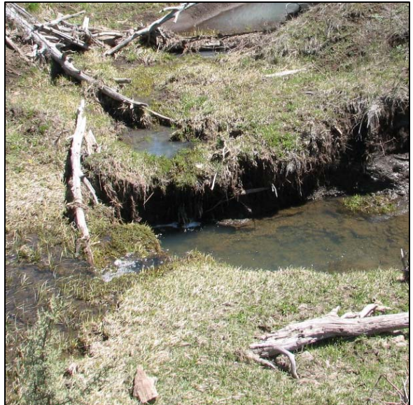
Figure 25. Headcut, viewed from upstream (Upper Klamath Basin, approximate channel width outside of the scour zone is 0.8 m). This is a medium-sized feature, given the channel dimensions.
