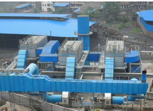
Figure 4. RTO installation at the DaTong coal mine in the Chongqing Province, China, (Photo courtesy of MEGTEC)
