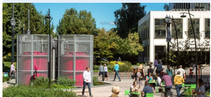
Hassalo on 8th Wastewater Treatment & Reuse System in Portland, Oregon — an example of an ONWS
