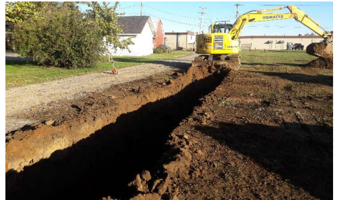
Photo #2: View looking north from MH #250055 during removal of old onsite VCP sewer lateral
