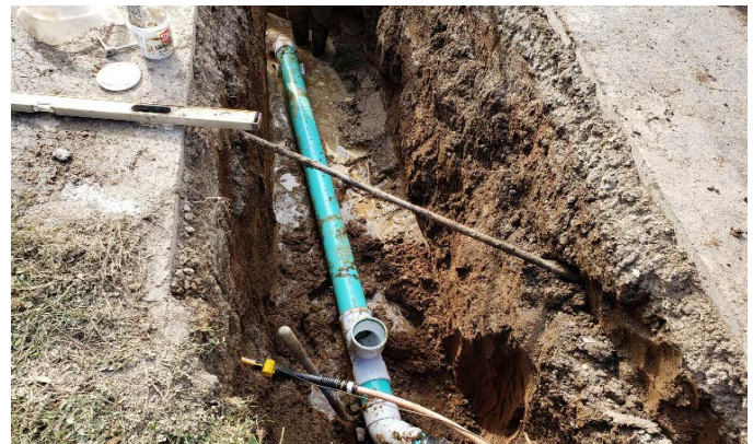
Photo #4: Looking west along new sewer lateral and cleanout for a residence
