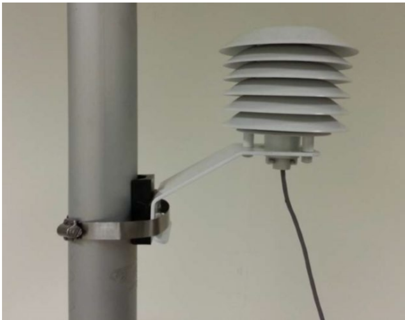
Figure 26. Ambient Temperature Probe Installed in Solar Shield
