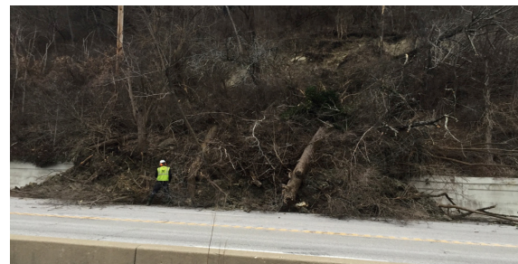
Figure 3. Destabilized Hillside on Columbia Parkway directly south of the site (City of Cincinnati Transportation and Engineering 2019)
