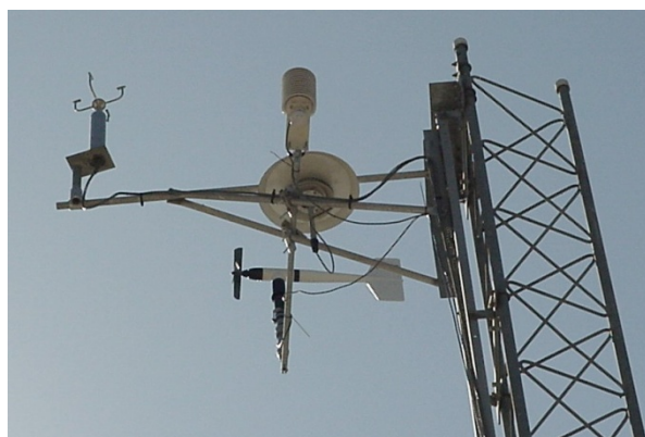
Figure 2.21 Typical Mounting of the Audit Sensors on the Site Tower
