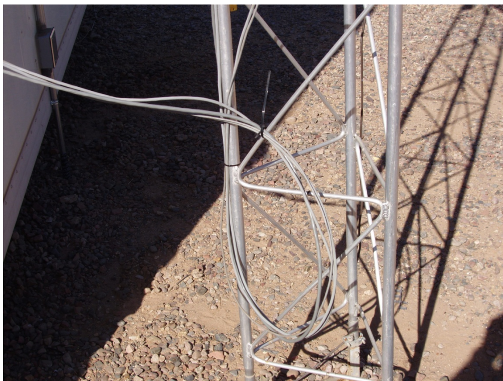
Figure 1.13 Signal Cable at Tower Base
