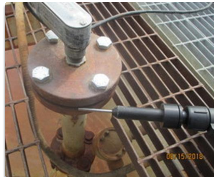
M21 Monitoring with a Flame Ionization Detector | Leaking level gauge
