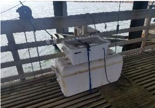
Coastal Bend Bays cooler system housing sensors
