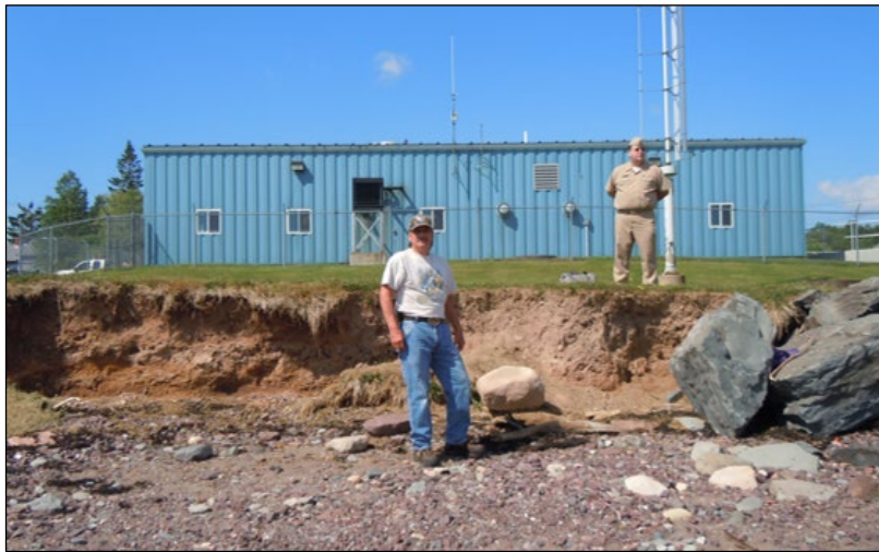
Image 4. June 23, 2016, Passamaquoddy Tribe – Pleasant Point eroding embankment – Gene Francis, WWTF Operator and Ken Grant, Indian Health Service engineer
