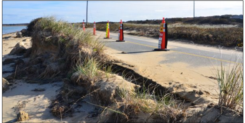
Image 3. October 29, 2012, Wampanoag Tribe of Gay Head (Aquinnah) Lobsterville Road Hurricane Sandy dune washout and road damage
