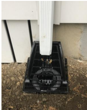
DOWNSPOUT SELF CLEANING GRATES
