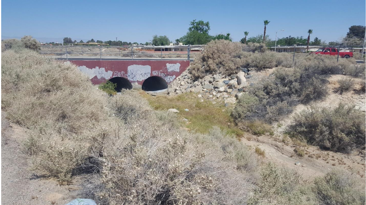
Figure 7. In Ridgecrest, CA, a culvert at an ephemeral stream crossing disrupts the movement of water, sustaining the growth of hydrophytes in the immediate vicinity. Photo credit: Cara Clark.
