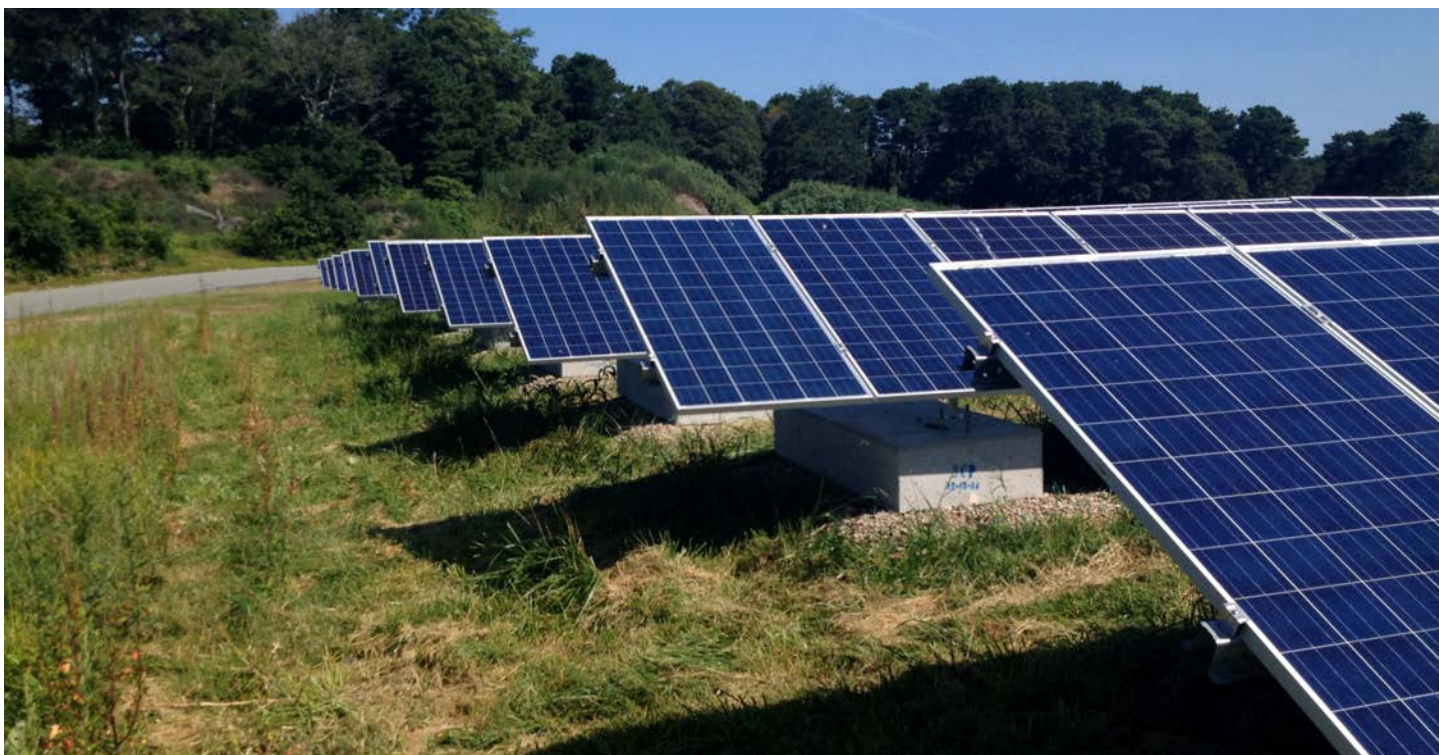
Figure 41: Solar panels. Photo by Weston & Sampson
