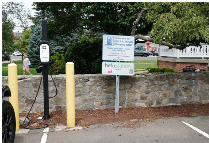
Existing Bridgeport EV Charging. Photo taken by MetroCOG.
