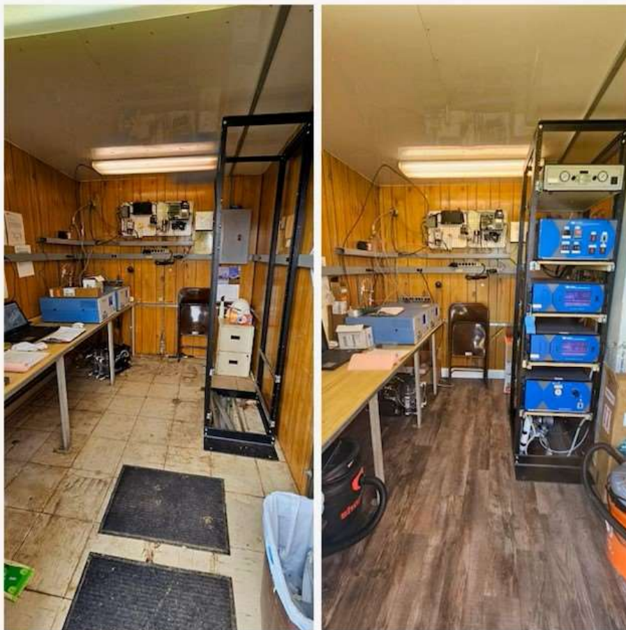
Figure 2 Stockton, IL (STK138) shelter before (left) and after (right) infrastructure repairs were completed (e.g replaced floors, sealed leaks inside the monitoring shelter, etc.).
