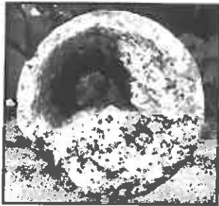
Grease clog in sewer pipe.
