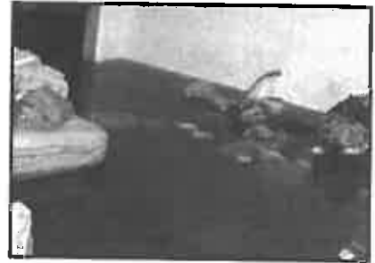
Sewer backup in residential basement.
