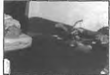
Sewer backup in residential basement.
