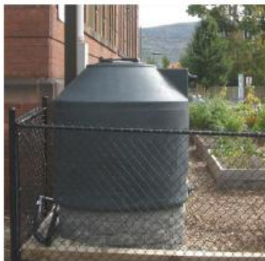
Cistern - Center Pepin Elementary School, Easthampton
